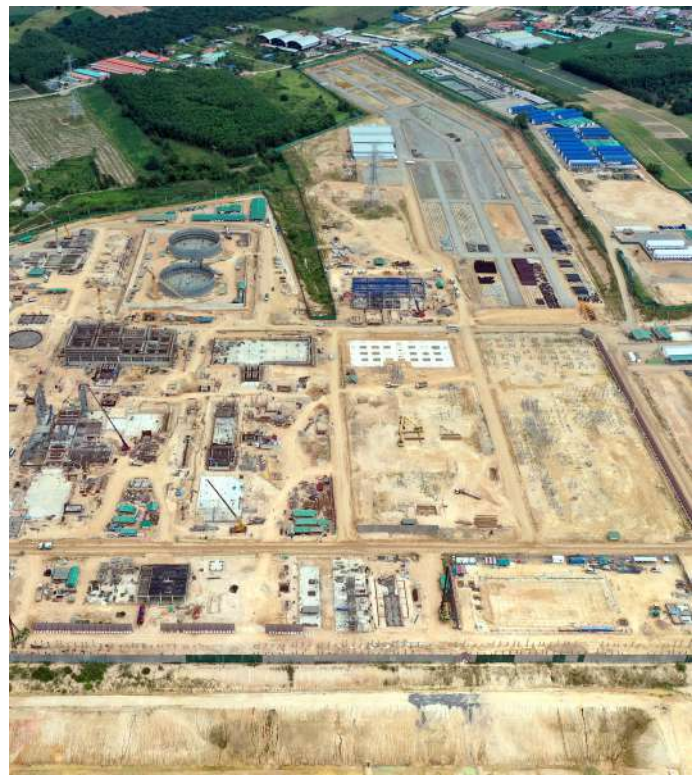
Power Block &amp; Balance of Plant Area
